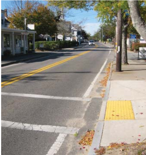
Curb ramp with slope and detectable warning strip on Route 28 in Harwichport.
