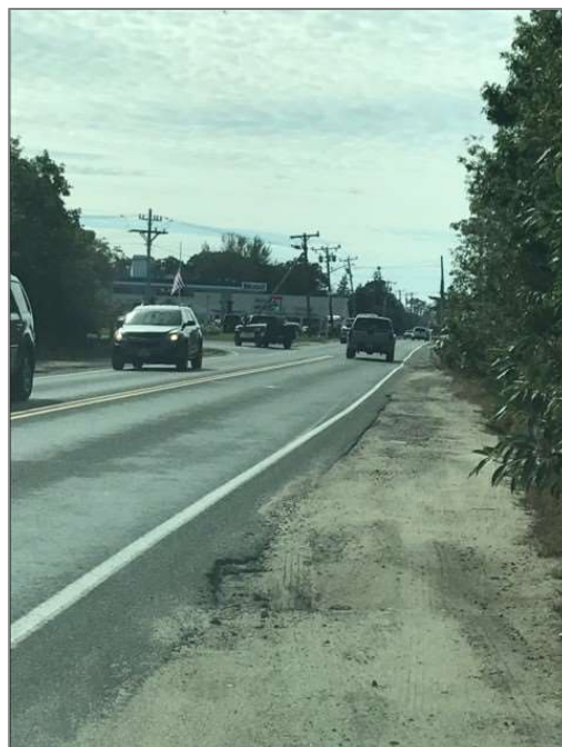
Figure 13. Yarmouth Road, Current Roadway Condition
